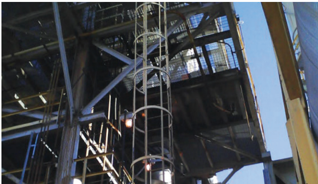
Before: Clearance, ladder, and cage hazards
